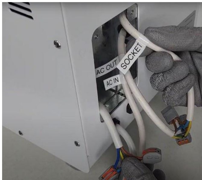
Image showing the cables and connectors inside the junction box
